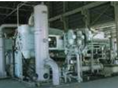
Process compressor for polyethylene
